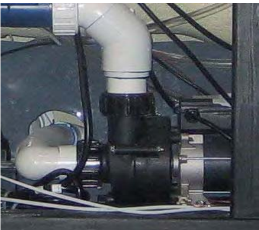
3) 24-hr Circulation pump
