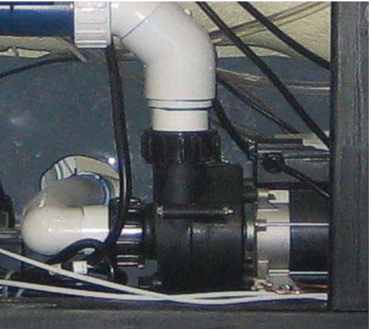
3) 24-hr Circulation pump
