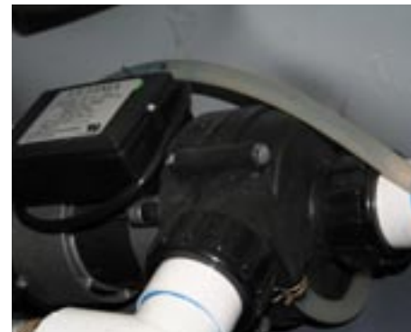
4) 24-hr Circulation pump
